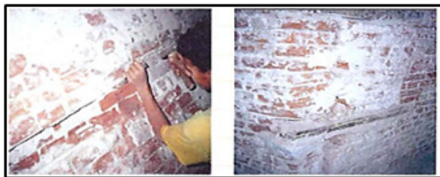
Fig. 20: Narrow, and deep crack after restoration [13] .
