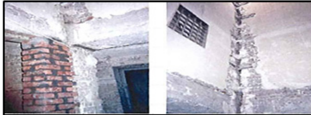
Fig. 19: Clarification of the crack in the entrance wall and the new brick shoulder [13] .
