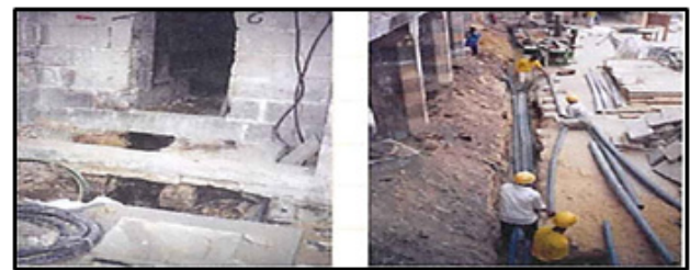
Fig. 23: New electrical distribution and installation [13] .
